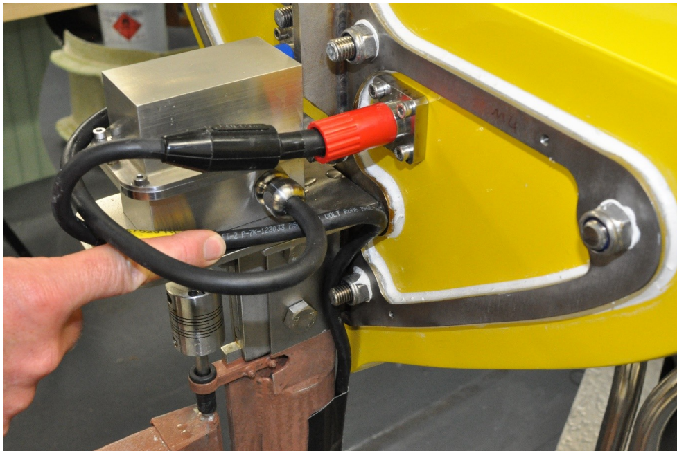
Figure 44 Stern rudder and POD cables in correct position before fitting stern cone
