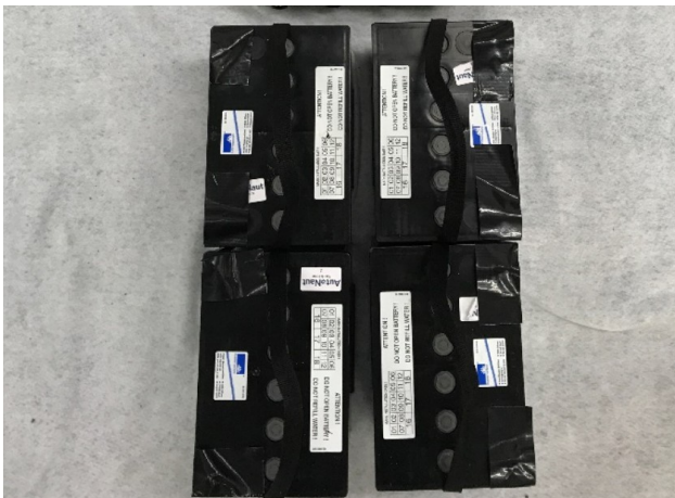
Figure 52 Bow batteries (left) Stern electronics (right)
